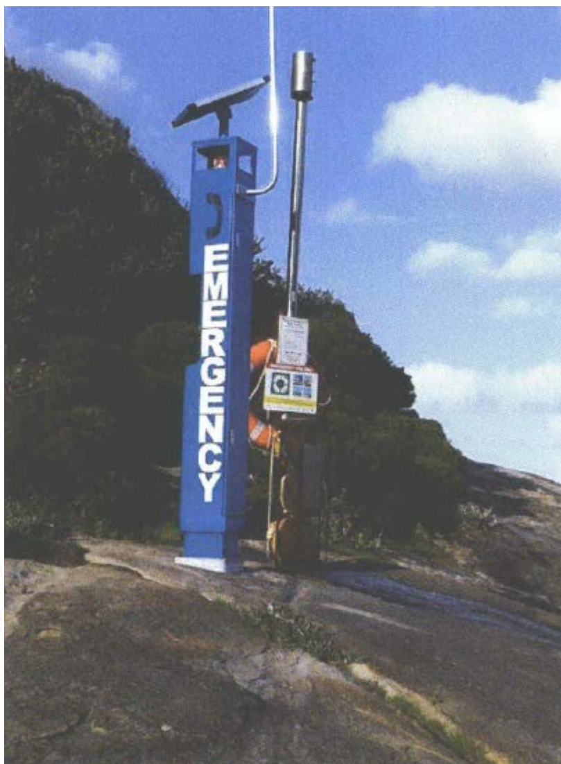
Exhibit 1, Tab 2, Page 10 – Emergency Phone Installed at Salmon Holes
